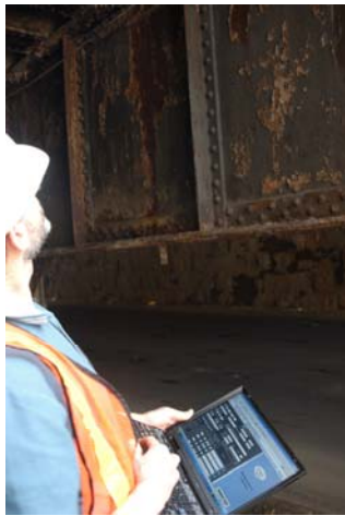
Ron Kovach of Wilbur Smith Associates uses the BridgeInspect™ Collector software in the field. Wilbur Smith Associates has conducted over 100 inspections using the software.
